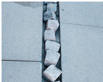
Looses Pflaster/Stolperfalle (Foto Jasmin Moor)
