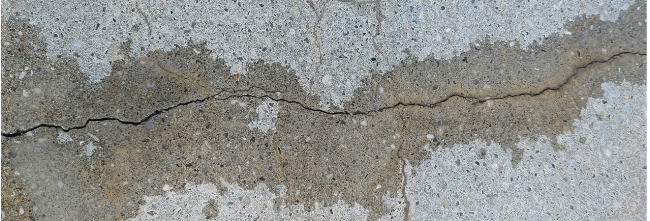
Figure 4-2: The appearance of the crack after spraying the solution of component A
