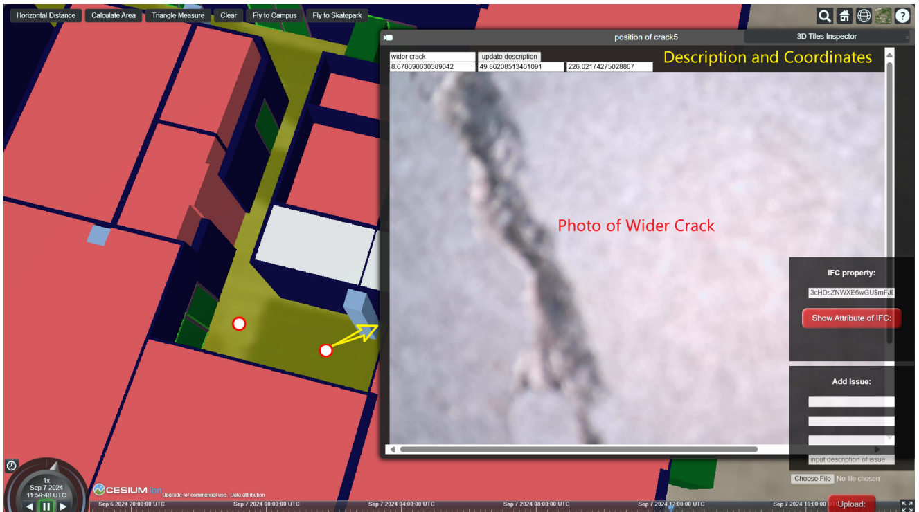
Figure 5-66: Visualization of wide crack and corresponding photo, description, and coordinates
