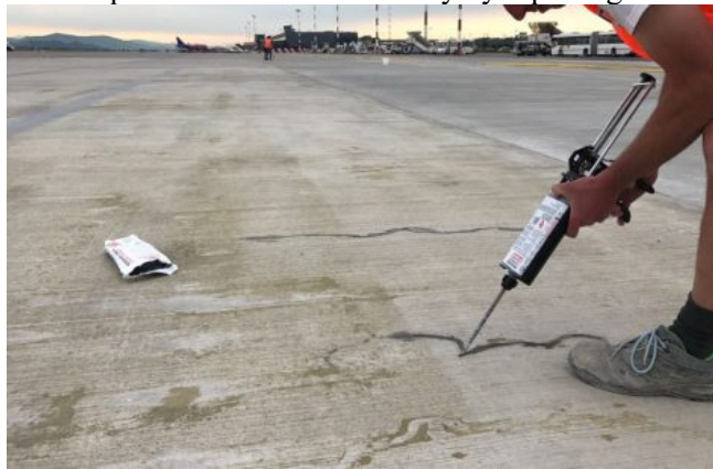
Figure 2-18: Crack repairs at Milan-Malpensa MXP International Airport using polyurethane injection (Glewwe, 2017)
