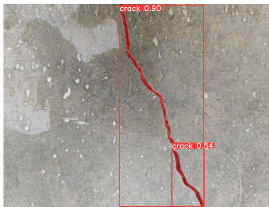
Figure 5-38: Crack segmentation result based on YOLOv8n in Jetson Orin Nano
