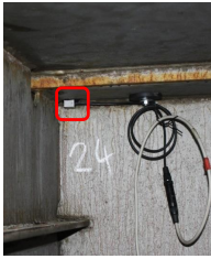
(a) installed sensor (photo: Hagen Berthold)
