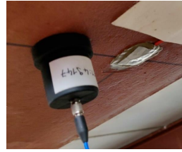
(b) installed acceleration sensor and strain gauge
