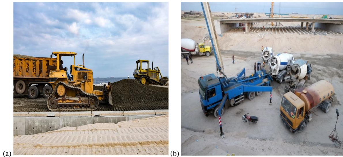
Plate 6.6[a and b]: Heavy-duty machinery utilised in the reclamation and construction of the EAC (Source: https://www.ekoatlantic.com/media/image-gallery/ )
