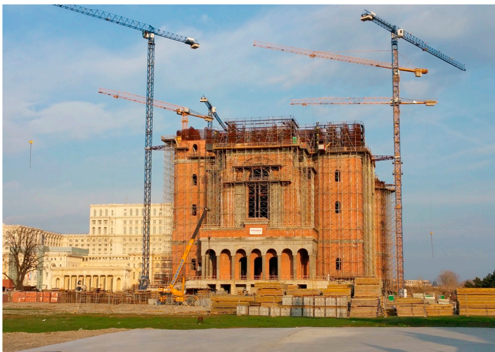
Figure 6. The construction of the gigantic People’s Salvation Cathedral in close vicinity of the Parliament Palace in Bucharest. Photo: Mirail Mihai, Creative Commons Attribution-Share Alike 4.0 International, https://creativecommons.org/licenses/by-sa/4.0/deed.en .
