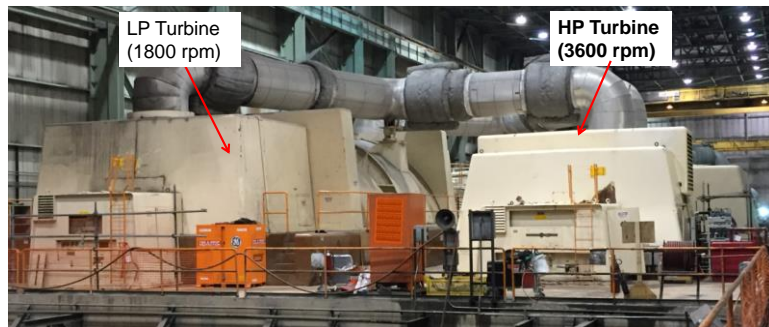
Figure 3: cross-compound steam turbine generator
