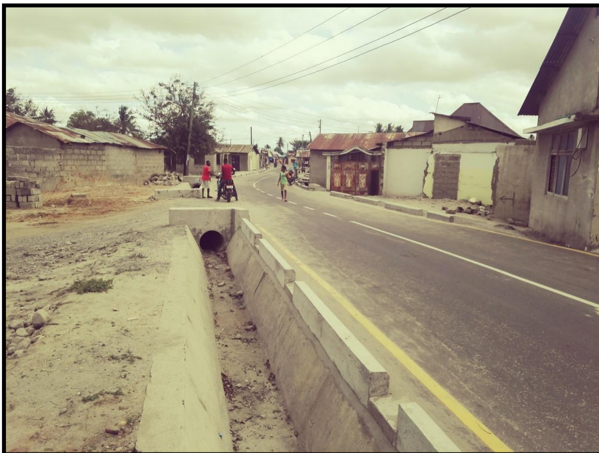
Figure 7.1: Surface Concrete Lined Drains on New Street Roads in Dar es Salaam Source: Photograph by Frank Edward (author) July 2017.
