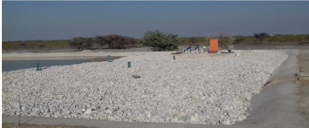
Figure 2.7: Rock filter installed in a maturation pond
