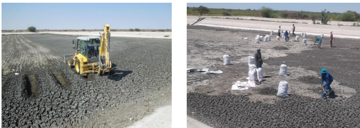
Figure 2.5: Removal of sun dried sludge from a facultative pond (left) and a maturation pond (right)
