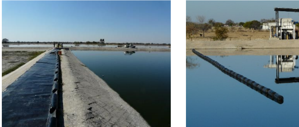
Figure 2.6: Preparation of floating baffle 1 (left) and baffle 2 installed in a facultative pond (right)
