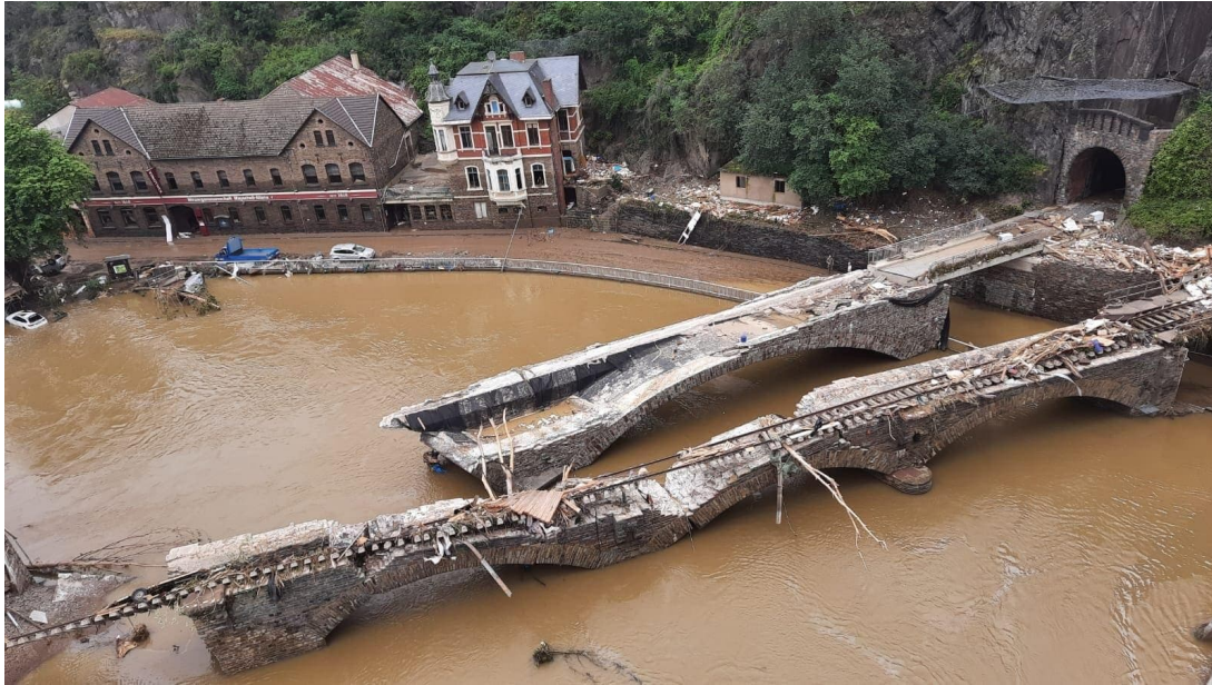
Figure 4.1: Destroyed bridges and flooded streets after heavy flooding in the Ahrtal, Germany. July 17, 2021 (Photo by Landespolizei Thüringen).
