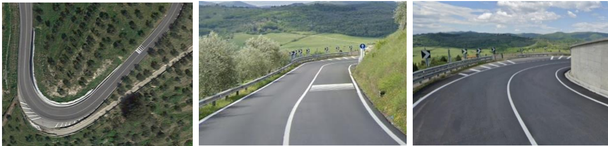
Figure 3.57 – Example of a critical curve, left - north oriented satellite view, right - photo approaching the curve from East. The curve is visible from distance but not understandable. The field of view shows many problems: the barrier line follows a different trajectory from the road axis, white markings along the shoulder create bad focus point and modify the perception of the road curvature (Andrea Paliotto, photos from Google Maps)
